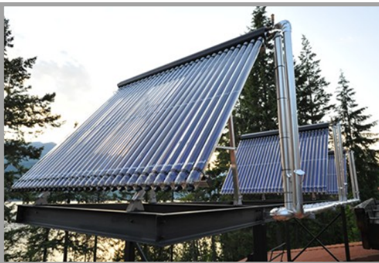
Solar Thermal panels at Yasodhara Ashram
